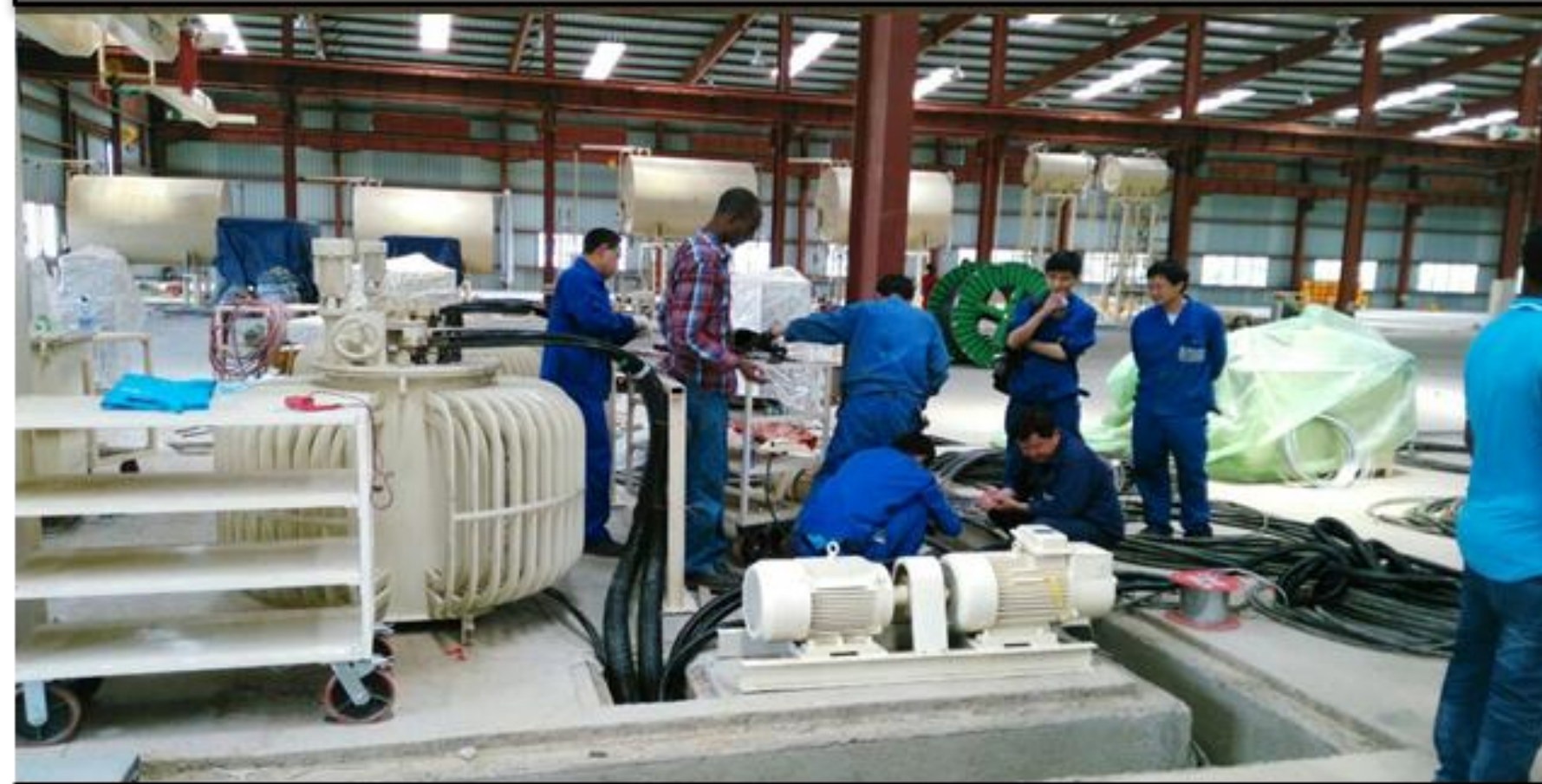
Site equipment debugging 2015
