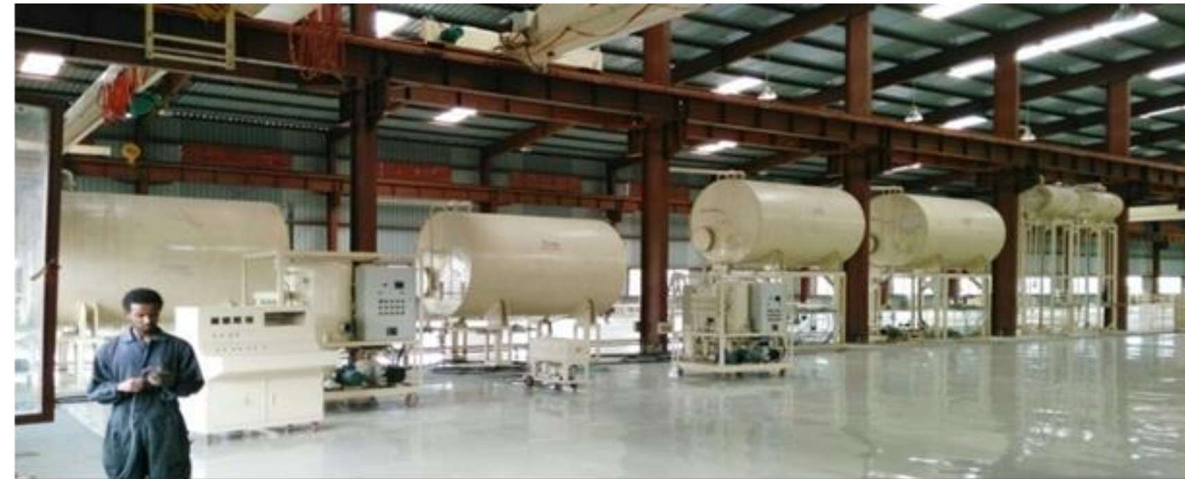
Transformer plant , indoor scene 2015
