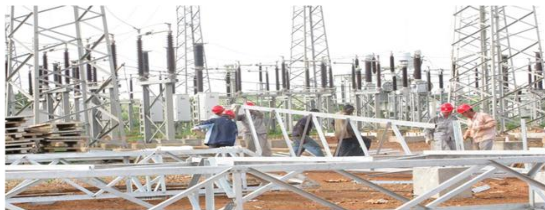
📍 154KV Transmission substation project 📅 2010
