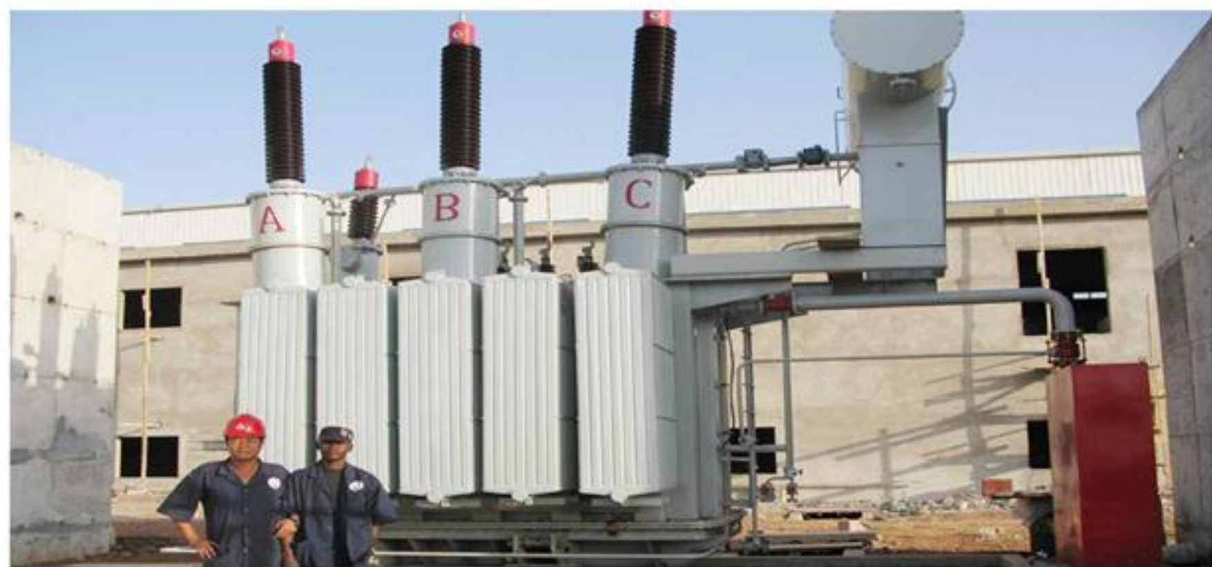
📍 2 × 4000KVA/154KV Substaion project 📅 2010
