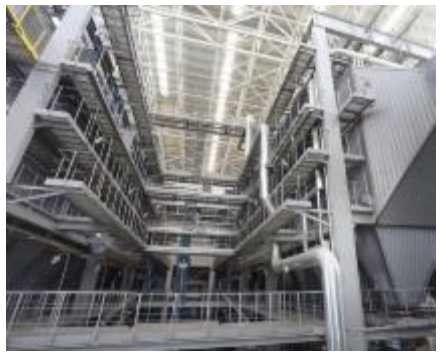
Flue Gas Cleaning System
