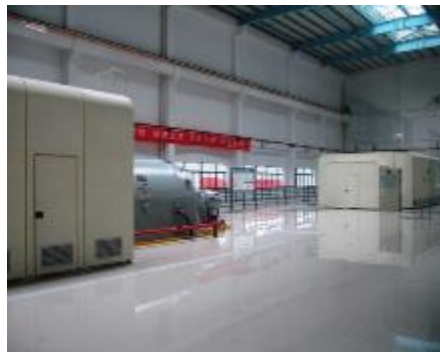
Turbine & Generator Room
