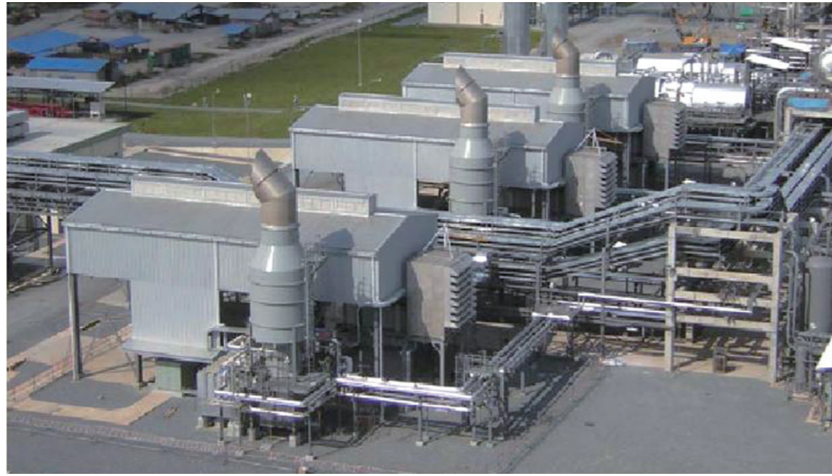
▪ Thermal Power Plant 热电厂
