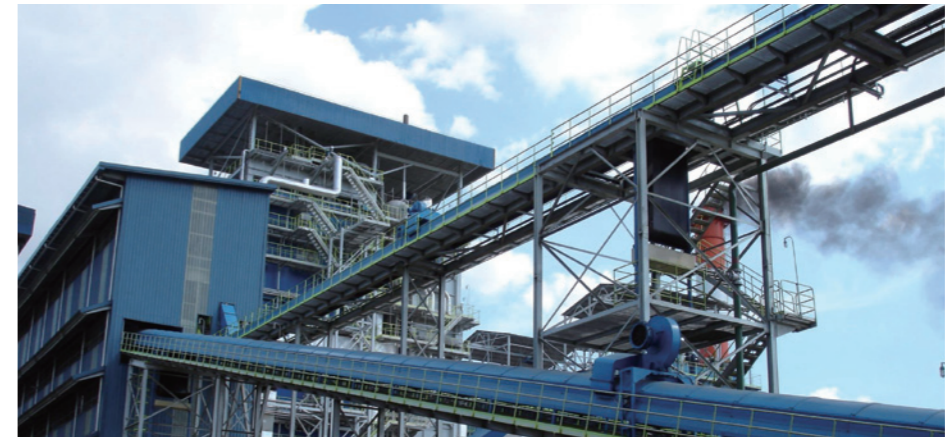
• Bagasse Conveying System and Boiler Workshop, Guyana Skeleton 8400TCD Sugar Complex
