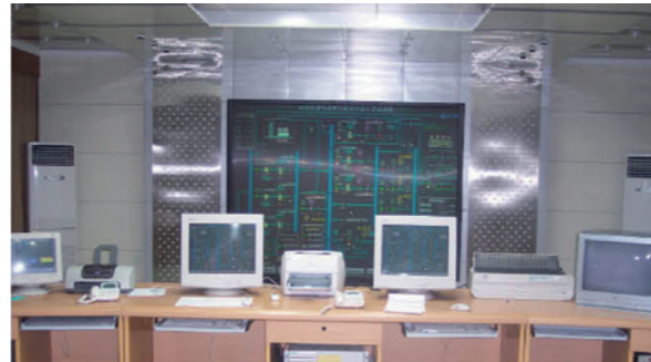
• Dispatching Station of Natural Gas SCADA System
